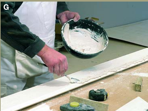
G Apply adhesive to the ceiling and wall areas of the cornice length
