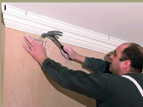
Press the cornice into its required position and fix the pre-nailed timber blocks
