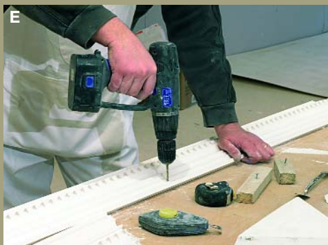
Pre-drill screw fixing holes in the cornice and counter sink for screw heads
