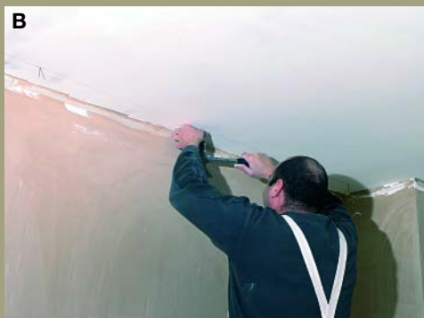
Fix nails along the chalk line as a ceiling guide for the cornice
